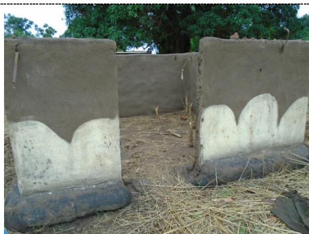
Fig 2. Shelter destructed due to crisis
