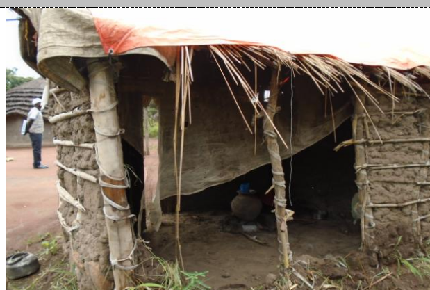
Fig 1. Destroyed occupied shelter
